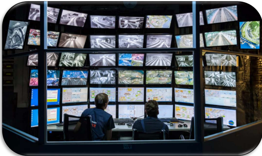
Figure 3.3 Control Room for traffic congestion and road surveillance.
