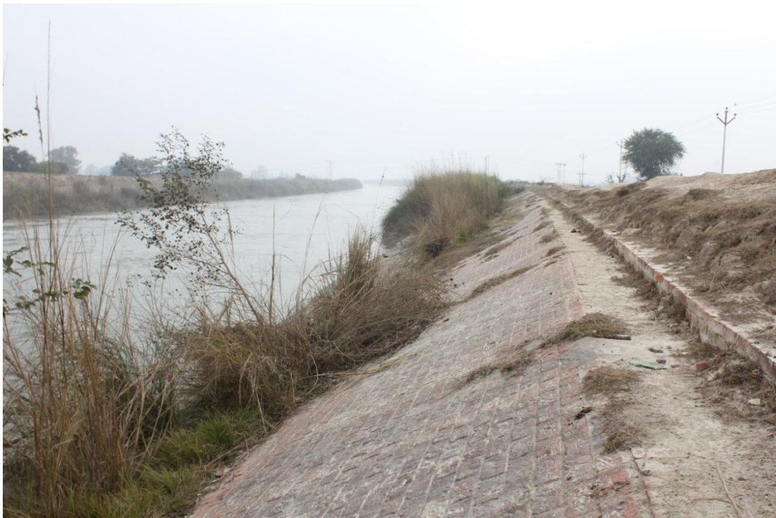
Improper lining of Canal (Elephant grass are grown)
